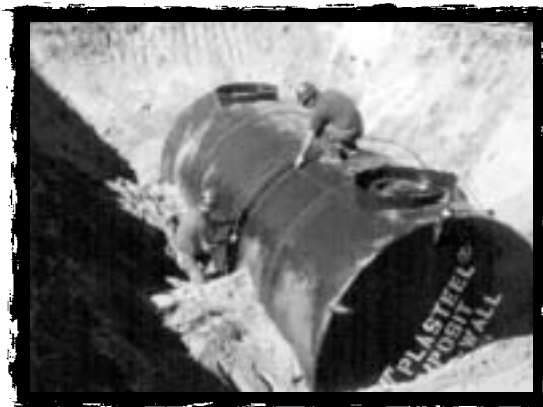
An offending Storage Tank unearthed.
