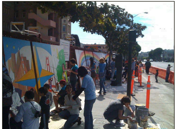
Top: After seven months of excavation, crews hit bottom on the two-story deep hole needed to complete the SFGH rebuild. That is enough dirt to fill a football field almost 60-feet deep! Bottom: Community members paint a mural that hangs along Potrero Avenue. The mural beautifies the area and helps conceal SFGH construction.
